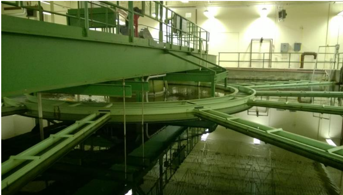
Solids Contact Clarifier
