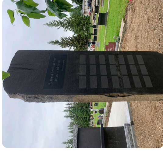
Figure 40: Memorial Wall, Lake View Cemetery, Cold Lake, AB (under construction). Source: LEES+Associates
