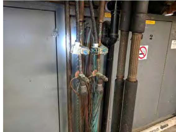
Figure 4-22 AHU-2 DX Coil Corrosion Visible
