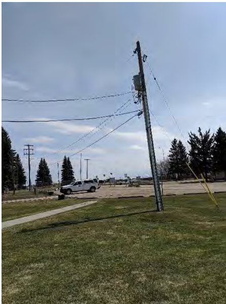
Figure 5-1 Utility Pole Mounted Transformer for West and East Wing Power
