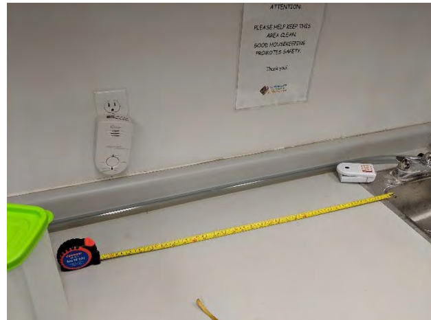
Figure 5-9 Receptacles Without GFI Protection
