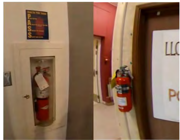
Figure 4-58 Typical Fire Extinguisher(s) - Both Semi-Recessed and Surface Mount Found
