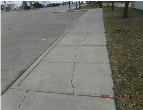
Figure 2-7 Parking Lot: Cracked Walkways
