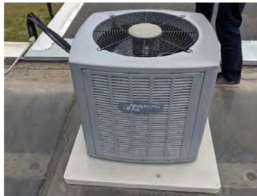
Figure 4-49 Newer Condensing Unit Serving the OTS Extension
