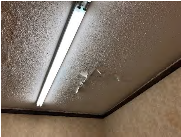
Figure 3-20 Water Damage to Richard Larson Ceiling
