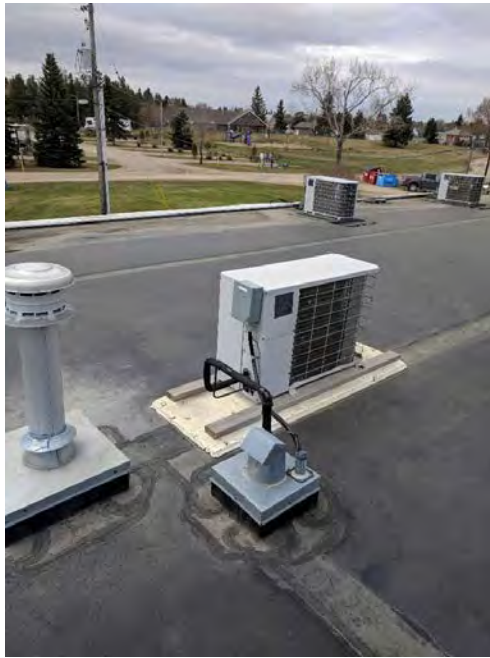
Figure 4-50 Condensing Unit Serving the Residential Portion of OTS
