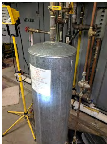
Figure 4-34 Glycol Storage Tank
