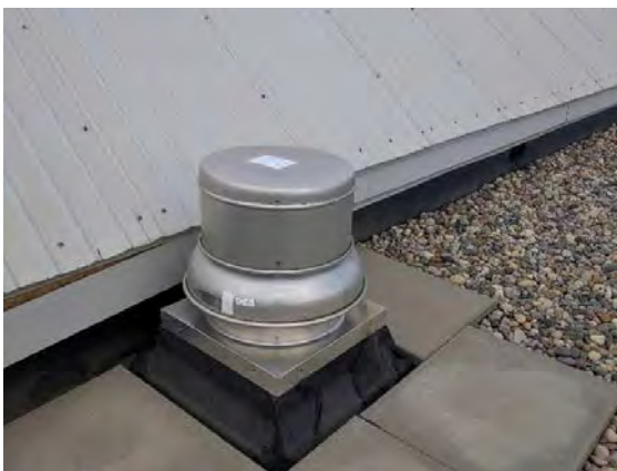
Figure 4-41 EF-1 on Roof
