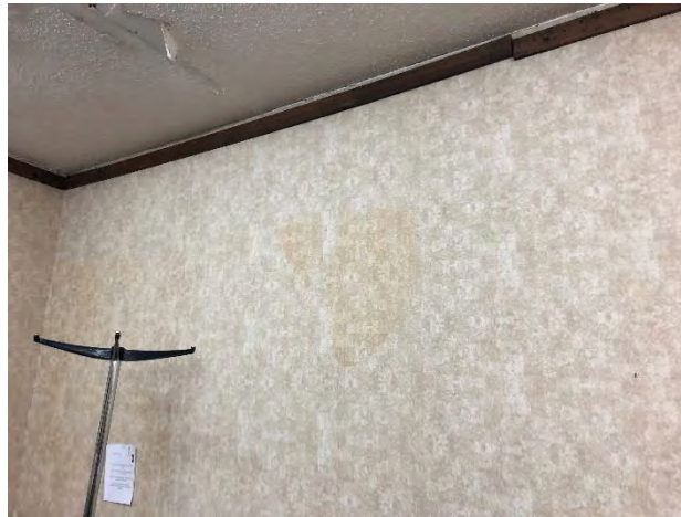
Figure 3-13 Water Staining on Richard Larson Wall
