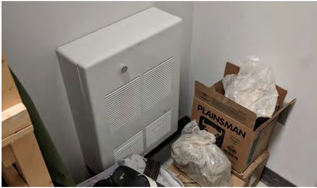
Figure 4-55 Electric Unit Heater in Pottery Closet
