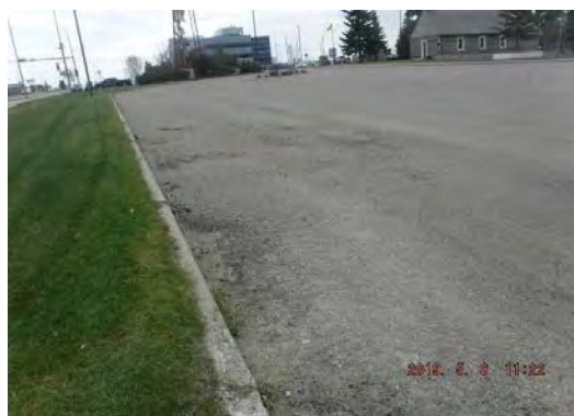
Figure 2-4 Parking Lot: Faded Road Markings
