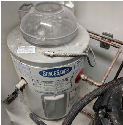
Figure 4-8 Electric Water Heater in the Kiln Room
