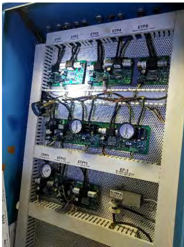
Figure 4-57 Pneumatic to Digital Control Panel
