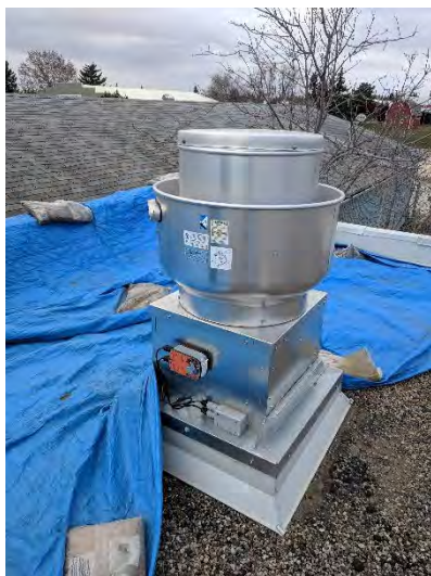
Figure 4-43 EF-2 on Roof
