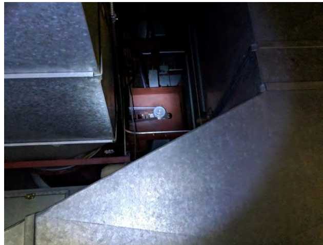
Figure 4-20 RF-2 Suspended From Roof, Not Easily Accessible
