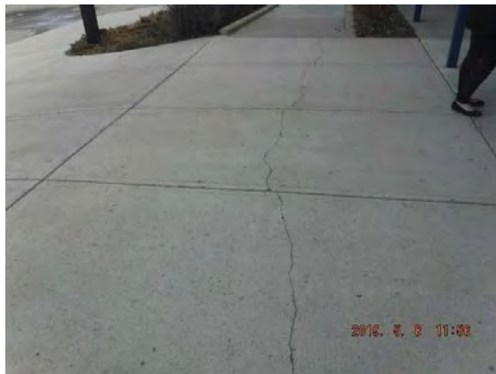
Figure 2-9 Cracked Concrete Pads
