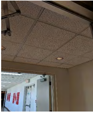
Figure 5-13 Vestibule Missing Smoke Detector
