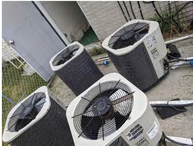
Figure 4-52 New OTS Outdoor Units (4 Units)
