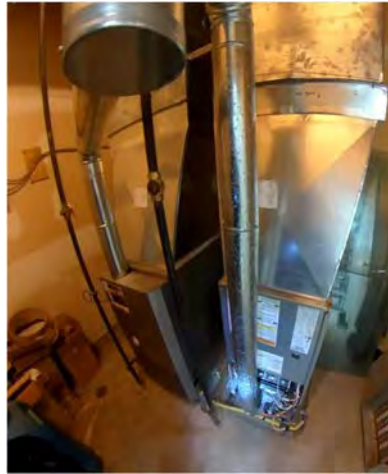
Figure 4-47 Richard Larson Mechanical Room with Payne Furnaces (Two Downdraft Furnaces)
