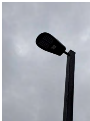
Figure 5-18 Parking Lot Lighting
