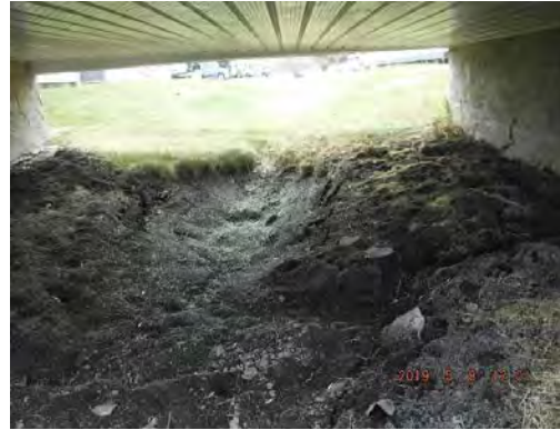
Figure 2-13 Eroded Swale Area Under Corridor
