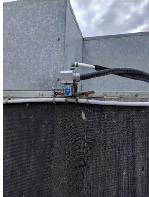
Figure 4-40 CH-2 Field Built Coil Water Cooling System
