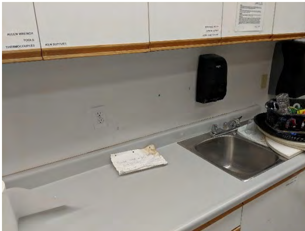
Figure 5-8 Receptacles Without GFI Protection
