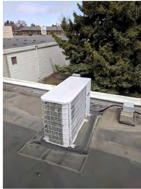
Figure 4-51 Typical Condensing Unit Near Edge of Building (not used anymore)
