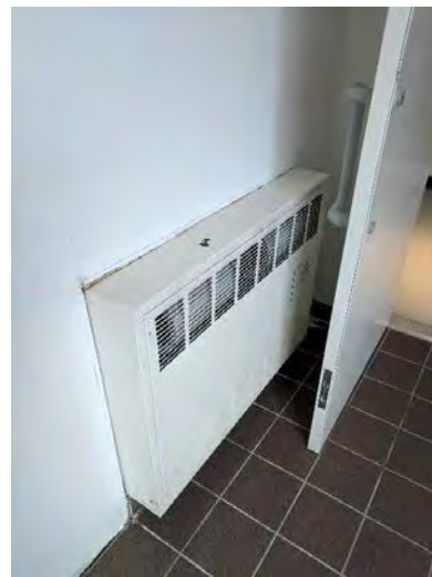
Figure 4-54 Original Cabinet Unit Heater in Corridor to Fuchs
