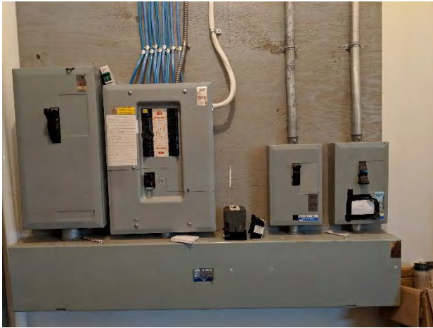
Figure 5-4 West Wing Main Distribution
