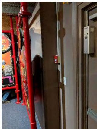
Figure 5-10 No Access to Main Disconnect for East Wing
