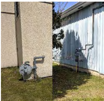
Figure 4-13 Cultural Centre/Richard Larson Gas Meter
