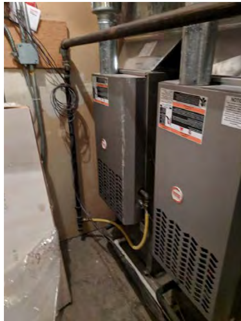
Figure 4-46 Typical Payne Downdraft Furnace Found in OTS Mechanical Room
