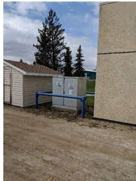
Figure 5-2 Pad Mounted Transformer for Main Museum Power
