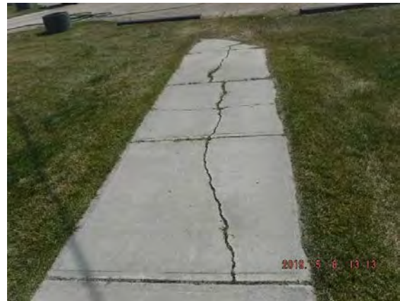
Figure 2-8 Rear Entrance: Cracked Walkways
