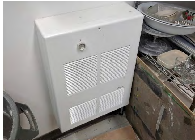
Figure 4-56 Electric Unit Heater in Kiln Room
