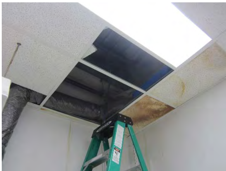
FIGURE 4 - Damage to Ceiling tile in Vault Area in BCHC due to Roof Leak
