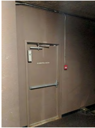
Figure 5-24 Missing Exit Sign
