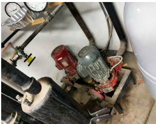
Figure 4-31 P1 and P2 System Pumps
