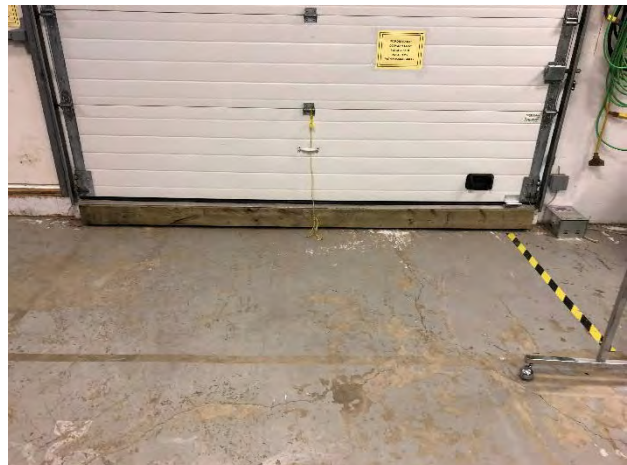
Figure 3-6 Typical Cracking in Richard Larson Slab
