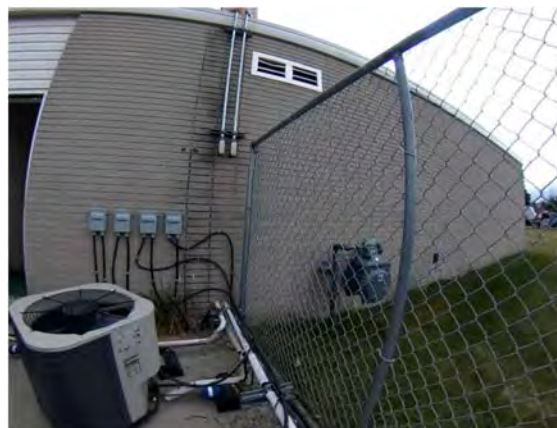
Figure 4-14 OTS Building Gas Meter
