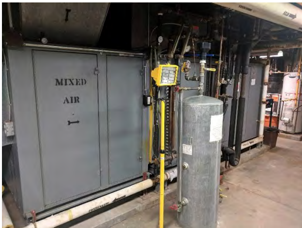
Figure 4-19 AHU-2 on Pad
