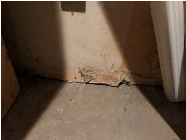
Figure 3-9 Viewing Water Damage in Heavy Oil Mechanical Room
