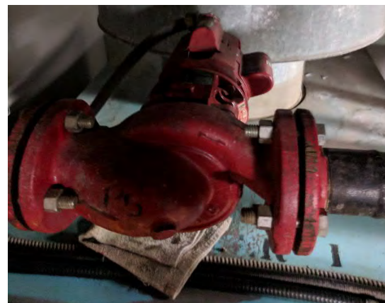
Figure 4-32 P5 Boiler Pump
