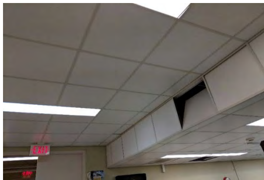
Figure 5-15 Missing Smoke Detector Higher Ceiling Area
