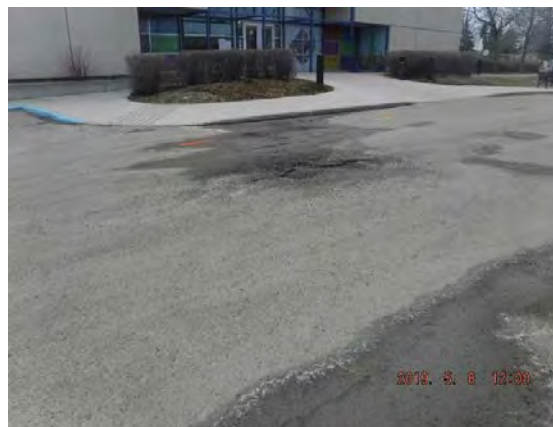
Figure 2-3 Parking Lot: Moisture
