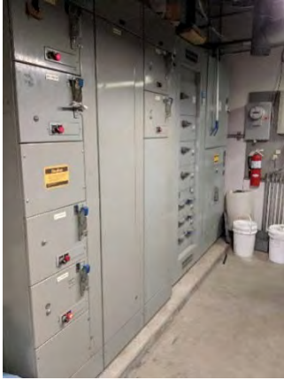
Figure 5-6 MCC and Main Distribution (Main Museum)
