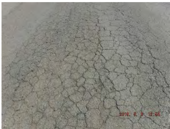
Figure 2-2 Parking Lot: Alligator Cracks
