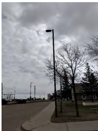
Figure 5-17 Parking Lot Lighting
