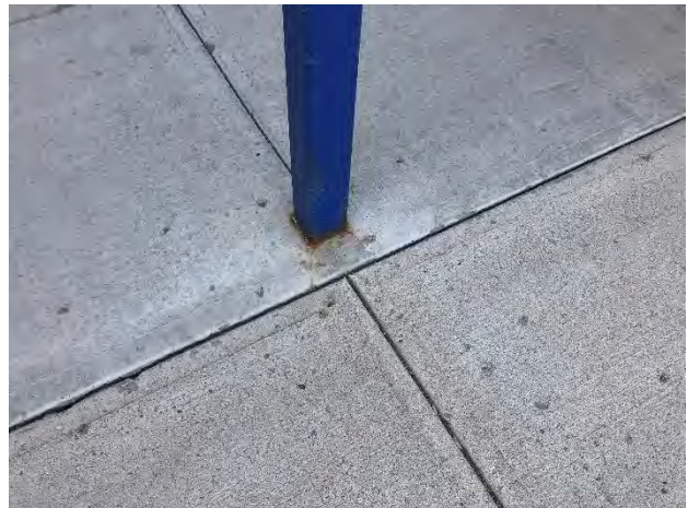
Figure 3-15 Viewing Corrosion at Bottom of Exterior Columns
