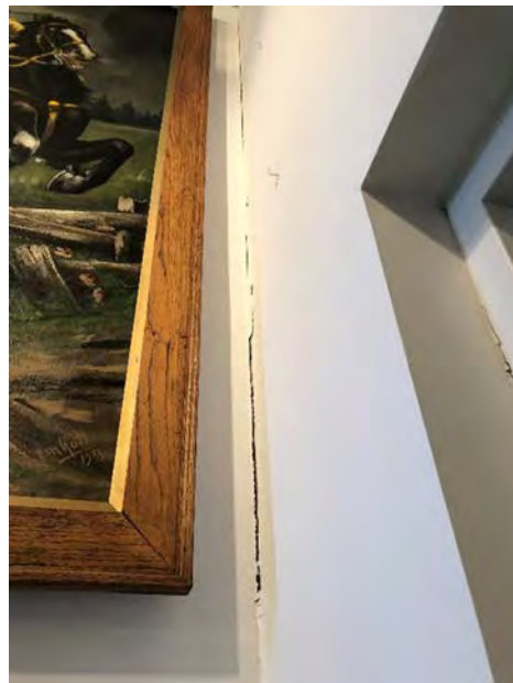
Figure 3-12 Viewing Crack in SE Corner of Imhoff Gallery
