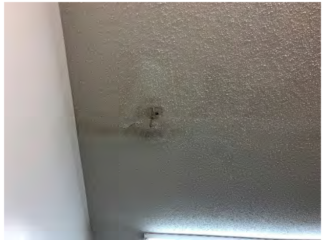
Figure 3-21 Water Damage to Richard Larson Ceiling
