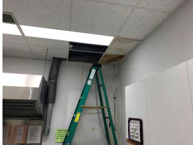
Figure 3-11 Viewing Water Damage in Link
