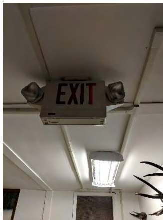
Figure 5-21 Exit Sign Barely Lit
