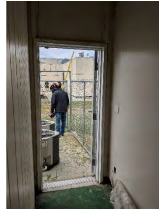
Figure 5-25 Missing Exit Sign
