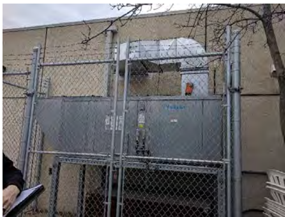
Figure 4-25 MUA-1 Outside Kiln Room
