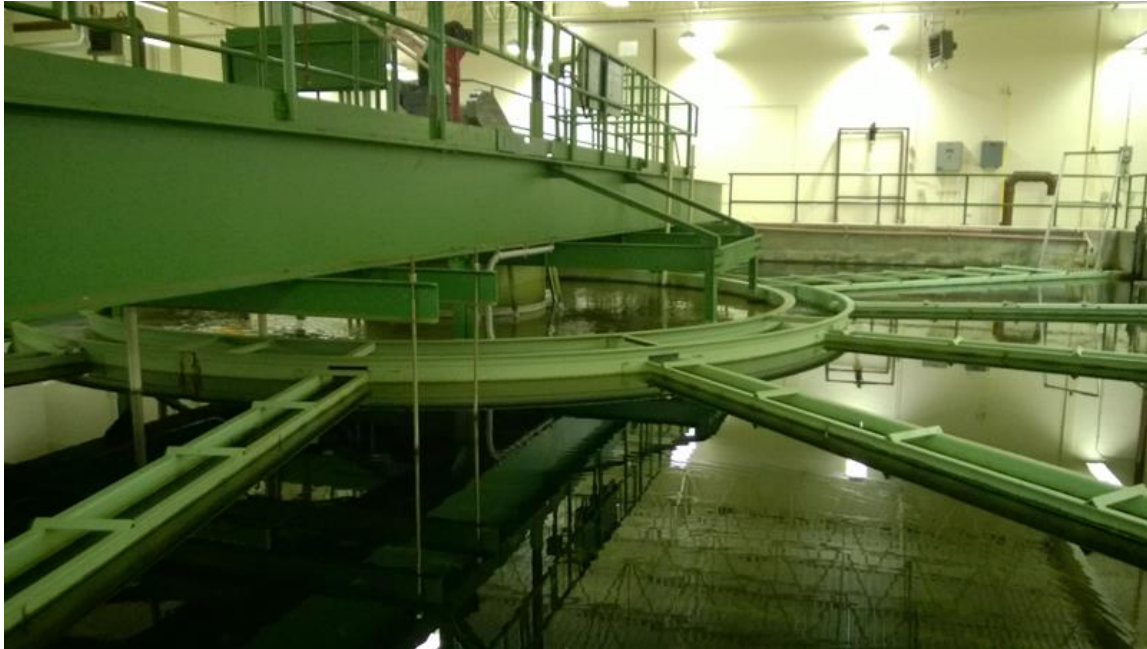
Solids Contact Clarifier
